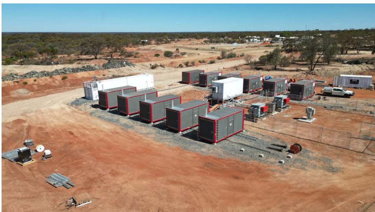
Figure 10 - Aerial view of primary power station.
