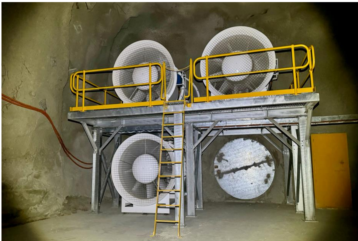
Figure 9 - Primary ventilation fans installed.
